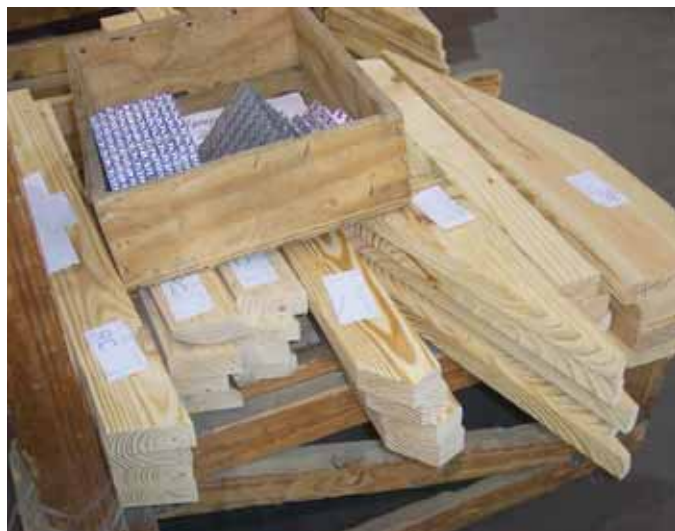
A box on top of cut webs contains the precise number of connector plates for that specific truss.
