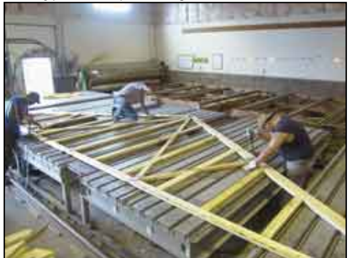
Studded structural gable being assembled on a steel topped gantry table. Notice the sound deadening blankets on the walls. Similar panels hang from the ceiling above
