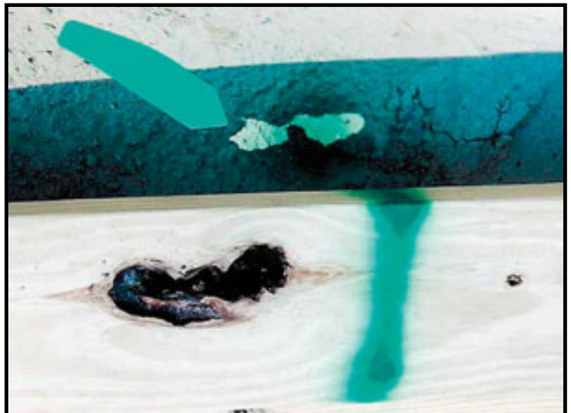
2X6 CHORD USING #2 LUMBER NOTICE SUNLIGHT THROUGH KNOT HOLE
