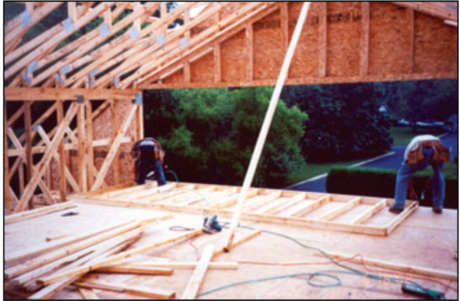
GIRDERS CARRY THE LOAD IMPOSED BY THE SECOND FLOOR AND ROOF ASSEMBLIES
