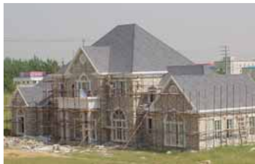
While this new construction might look like a typical Western home from the outside, the Chinese do not sell homes with fixtures and appliances in place. These are the responsibility of the homebuyer.
