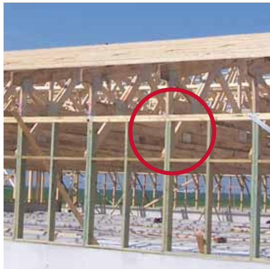
Figure 1. Knee brace used on an agricultural building.
