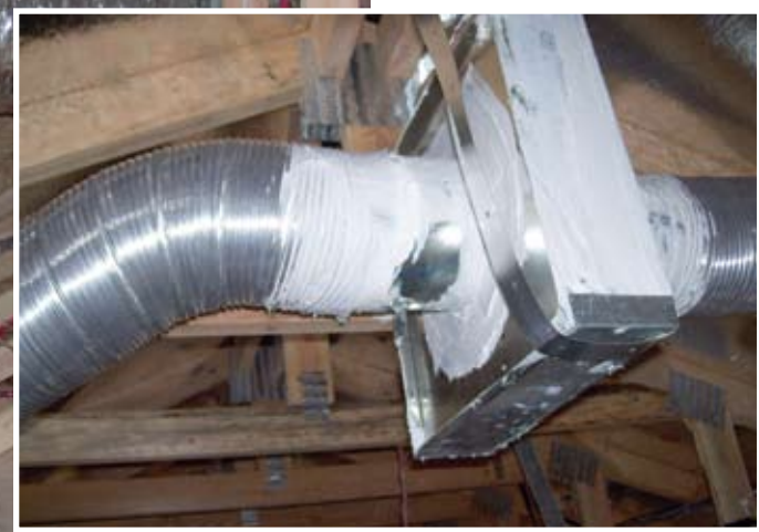
Raised heel trusses provide additional space for fresh air ducting. Outside air passes through a filter, circulates through this mechanical system and into the house.
