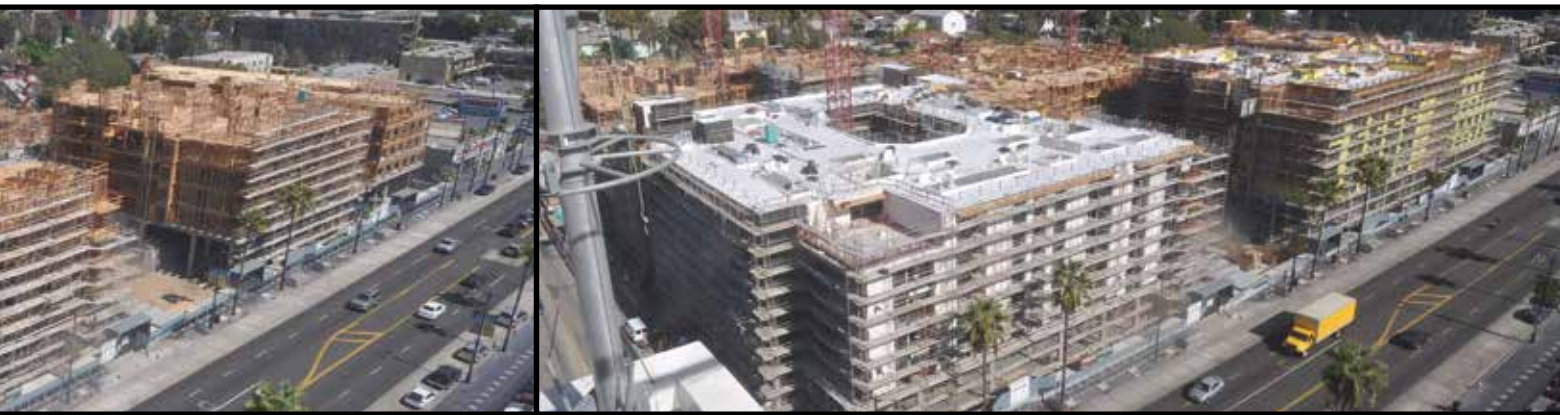
materials and framing labor. The amount of jobsite waste was dramatically reduced, and the buildings will be completed far ahead of schedule.
